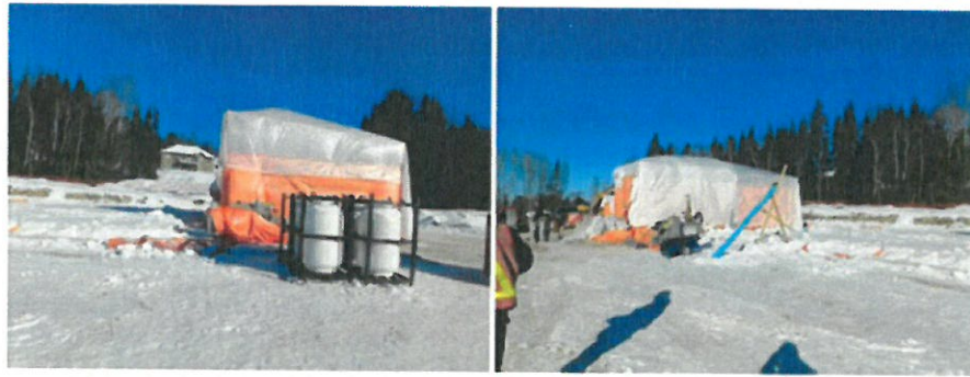
Protective enclosures at stairwells and elevator hoist way provide heat and weather protection to lay concrete block
