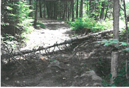
Another unpassable section of the trail.
