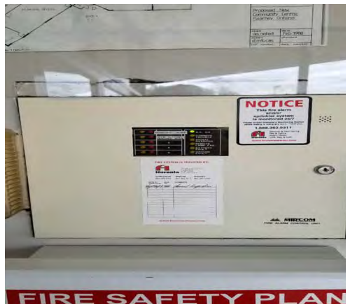
EXISTING MAIN FIRE ALARM CONTROL PANEL
