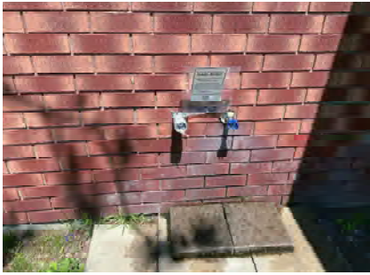
EX010 - Municipal Office Public Water Filling Station
