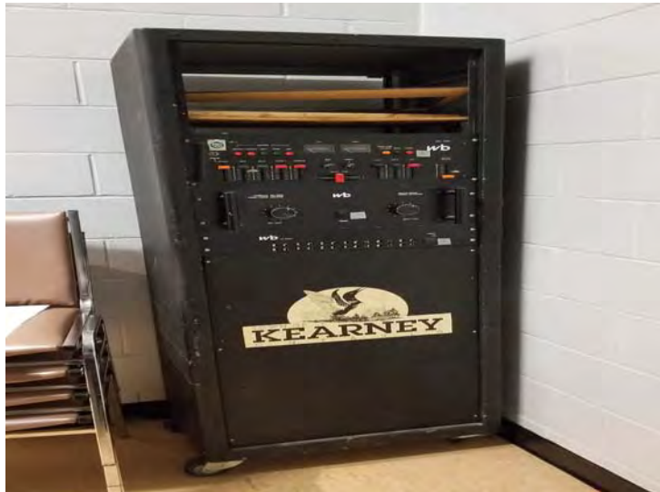
EXISTING LOCAL SOUND SYSTEM RACK AT THE STAGE OF THE GYM
