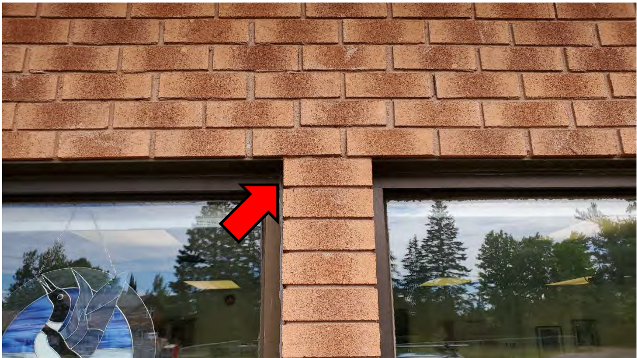
Figure 24: Community Hall Addition: Cracked bricks at lintel bearing.
