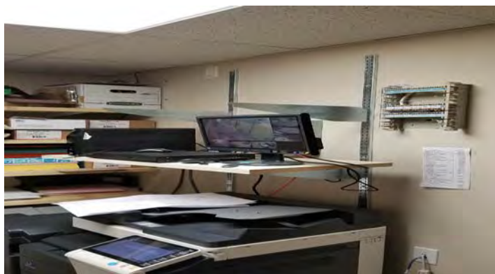
EXISTING CCTV SYSTEM AT THE FILE ROOM WITHIN THE OFFICE AREA
