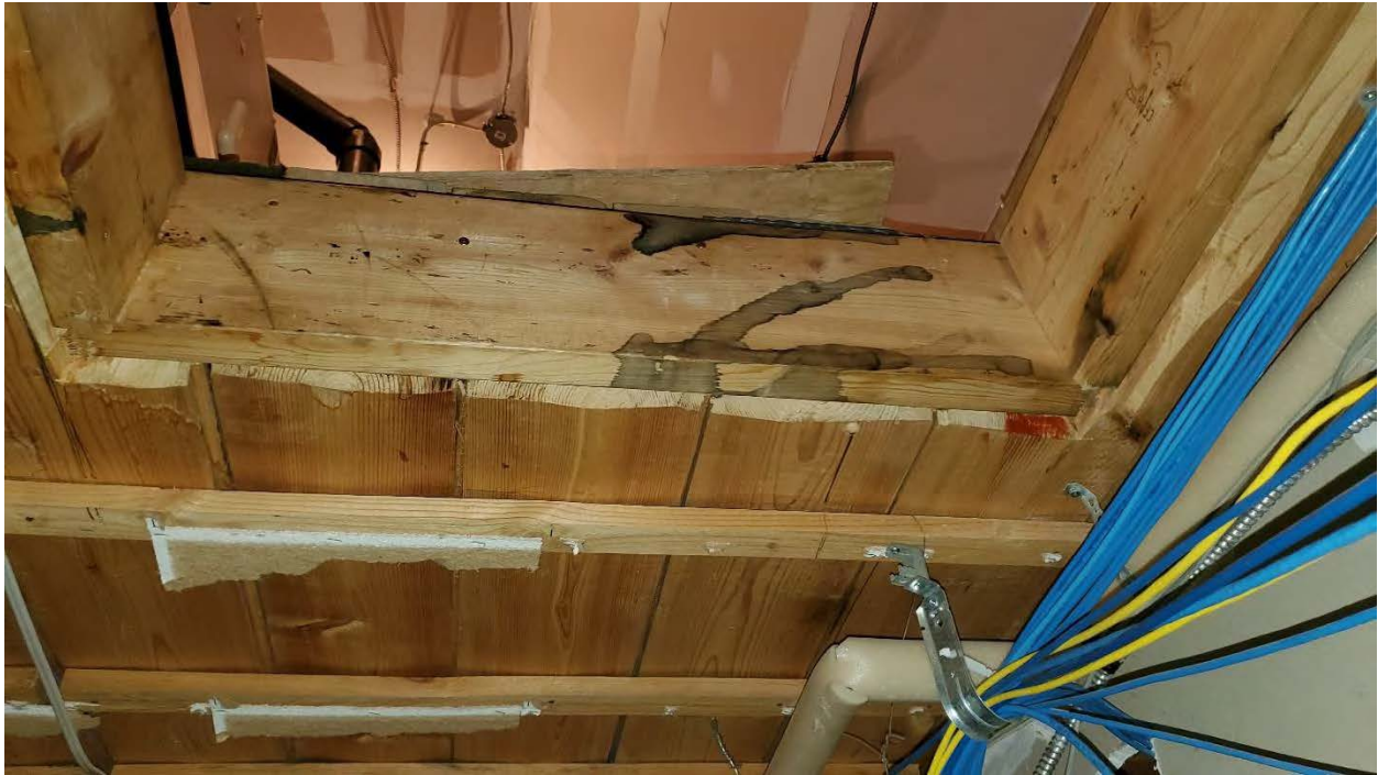
Figure 5: Municipal Office: Unsupported wood plank decking at Loft opening.
