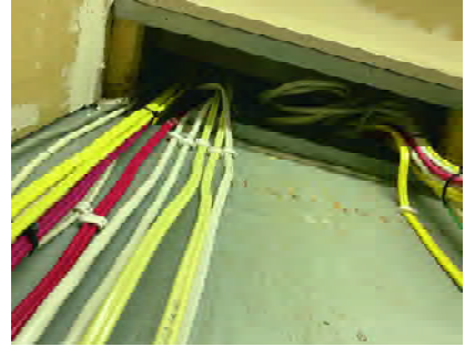
INT030 - Electrical Room Electrical Chase
