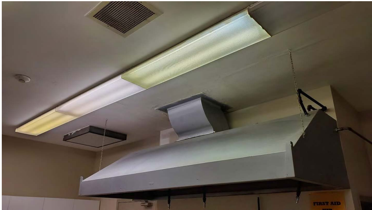
Figure 15: Community Hall Addition: Location of previous roof leakage in the Kitchen.
