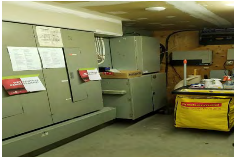
EXISTING MAIN POWER DISTRIBUTION SYSTEM AT THE MAIN ELECTRICAL ROOM
