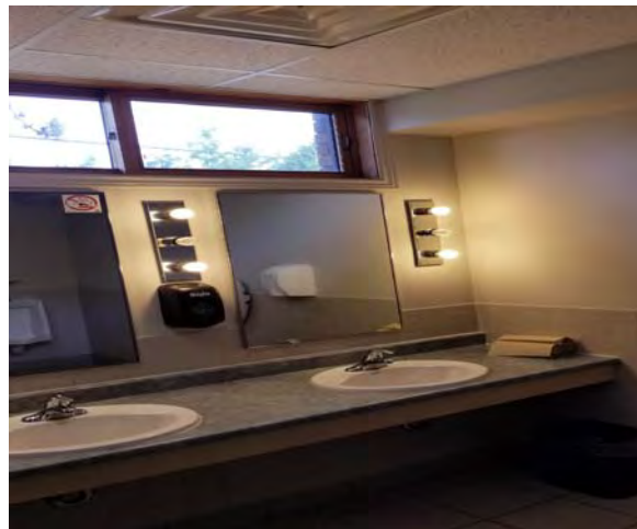
PICTURE OF WASHROOM FIXTURES
