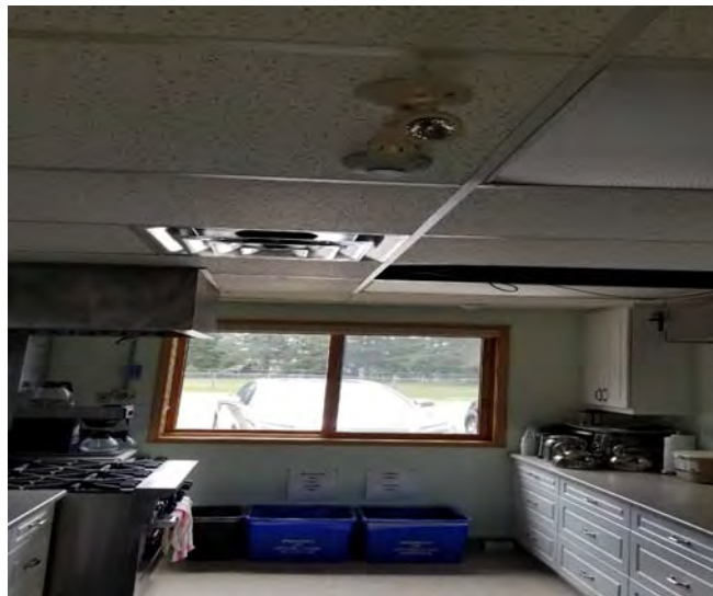
EXISTING EMERGENCY LIGHTING
