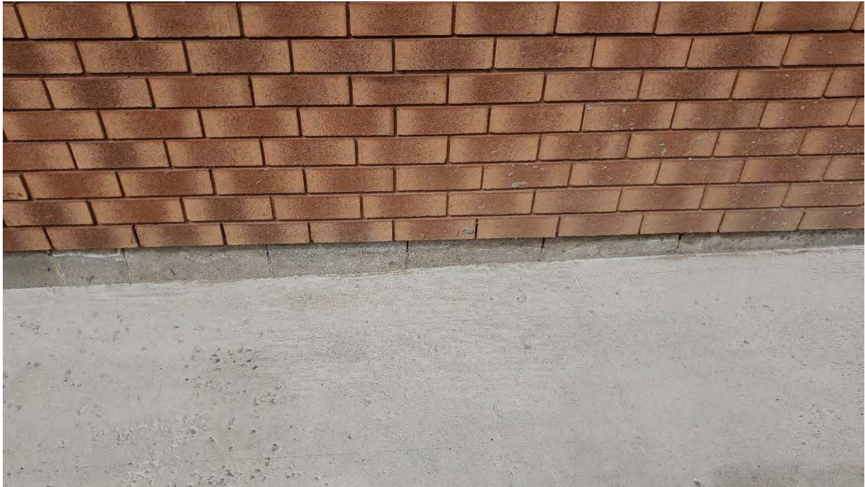
Figure 25: Community Hall Addition: Cracked mortar joints in the foundation wall on the east elevation.
