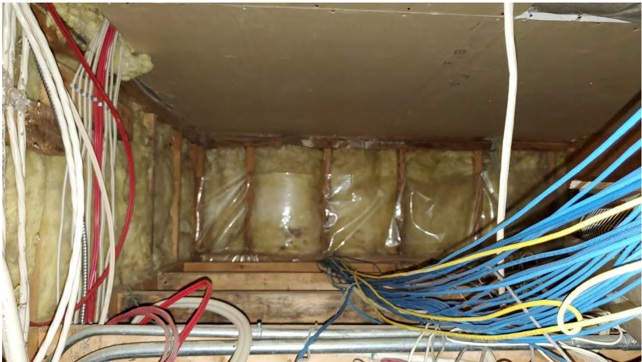
Figure 20: Electrical Room Addition: Wall framing above the ceiling in the Electrical Room.
