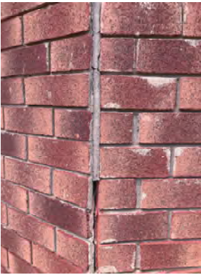
EX047 - Senior Club Main Entrance Brick Corner
