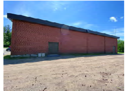
EX024 - Community Hall West Gymnasium Wall
