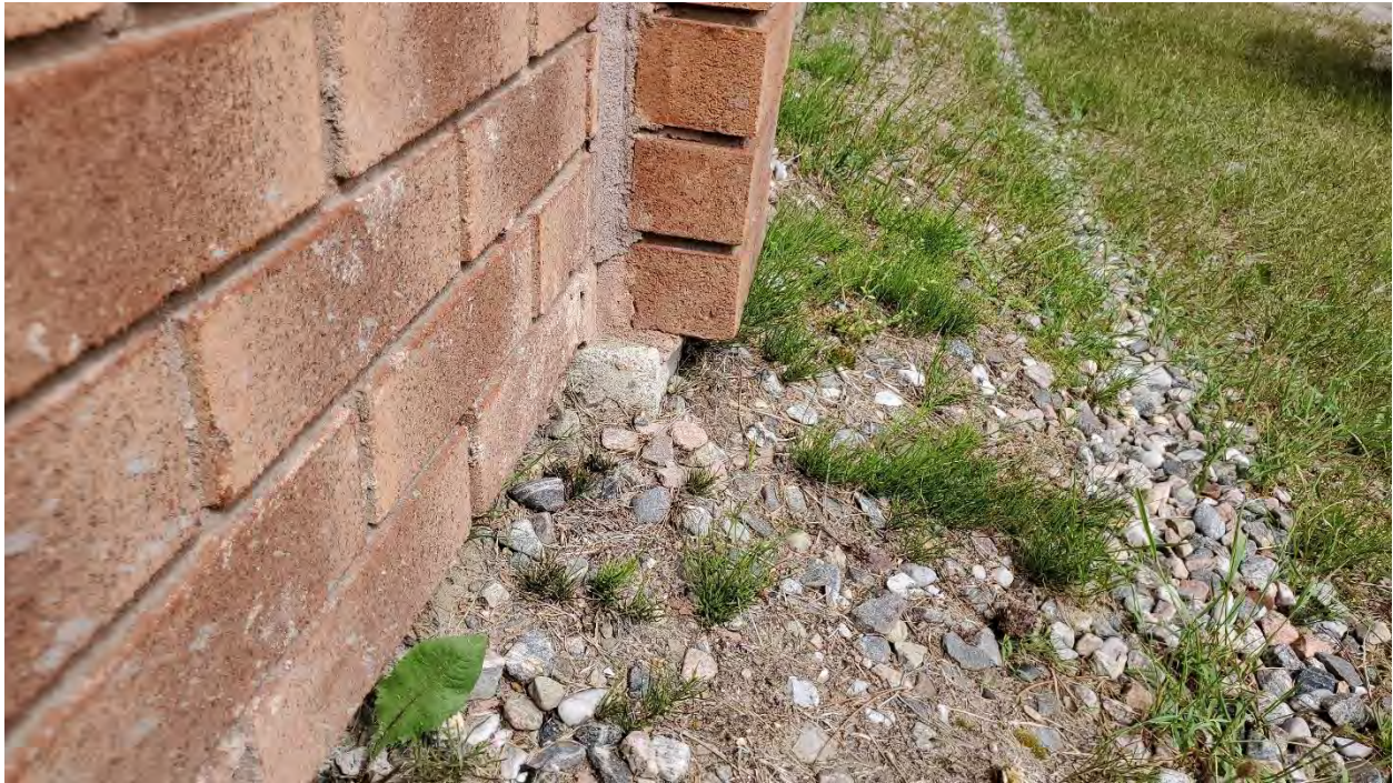
Figure 17: Community Hall Addition: Excessive brick projection beyond the foundation wall on the east elevation.
