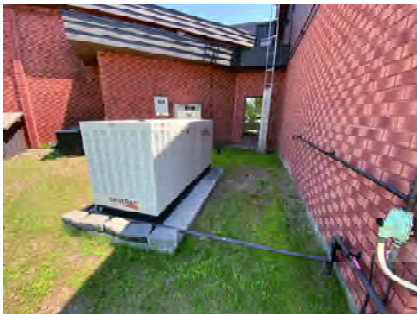
EX016 - Municipal Office Mechanical Exterior Alcove
