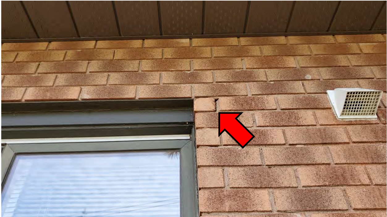
Figure 7: Municipal Office: Loose brick at lintel bearing on west elevation.
