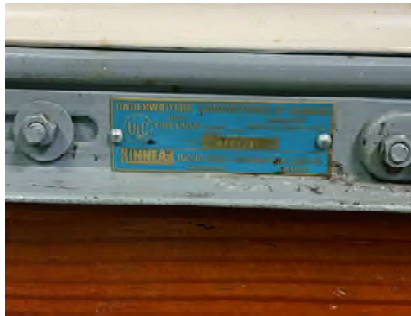
INT013 - Bar Fire Shutter Rating Label
