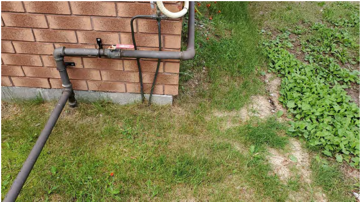
Figure 10: Municipal Office: Excessive brick projection beyond the foundation wall on the west elevation.
