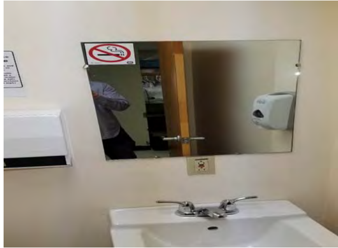
PHOTO OF PLUMBING FIXTURES (WASHROOM ACROSS THE GYM)
