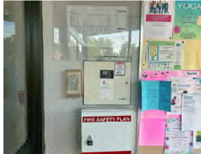
INT110 - Vestibule Annunciator Panel
