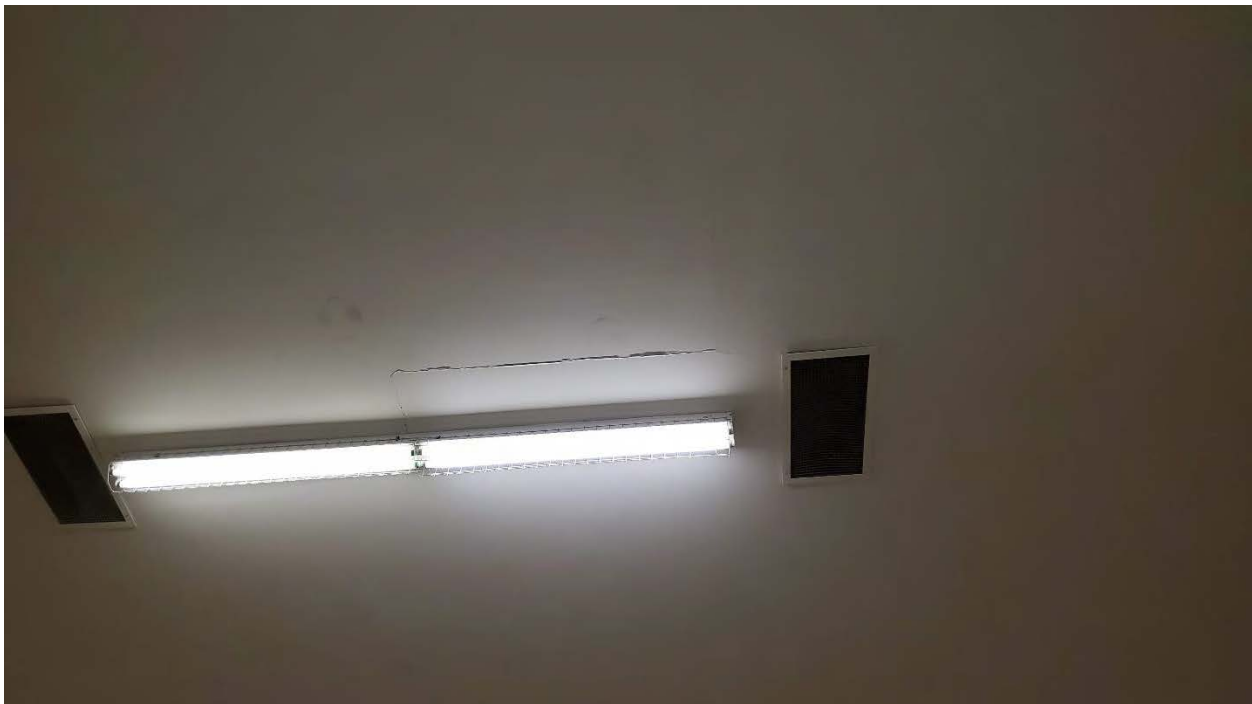
Figure 14: Community Hall Addition: Ceiling crack over Gymnasium.
