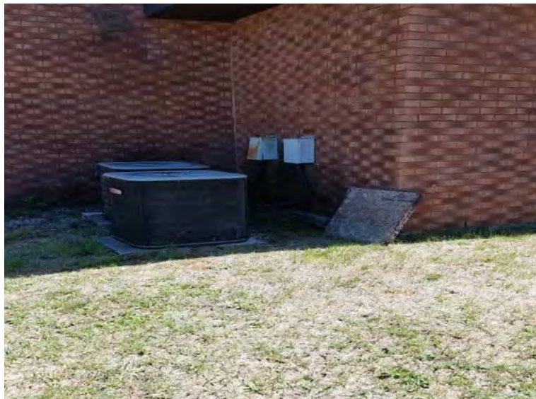
PHOTO OF CONDENSING UNIT (SERVING SENIOR'S CLUB AND OFFICE)
