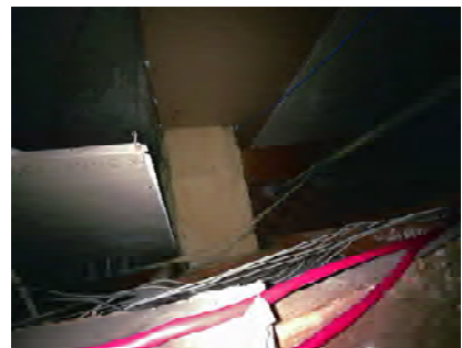
INT027 - Electrical Room Ceiling Plenum looking East
