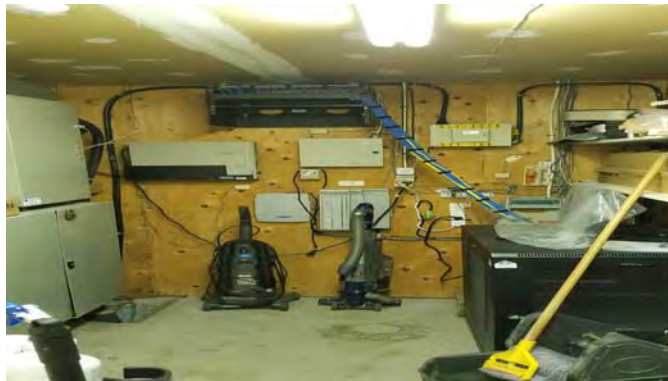
EXISTING INTRUSION ALARM CONTROL PANEL, TELEPHONE SWITCH AND IT CABINET LOCATED AT THE MAIN ELECTRICAL ROOM
