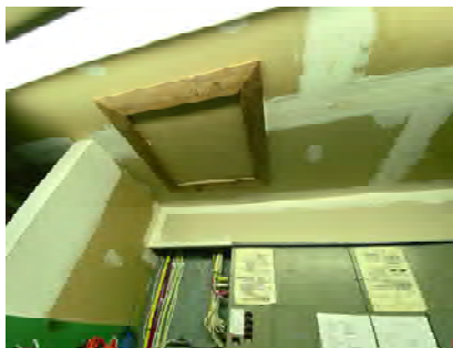
INT025 - Electrical Room Ceiling Access Panel
