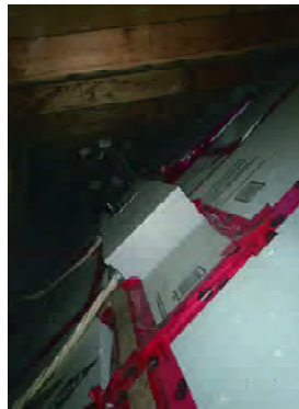
INT005 - Gymnasium Attic Space Mech Unit Electrical Panel
