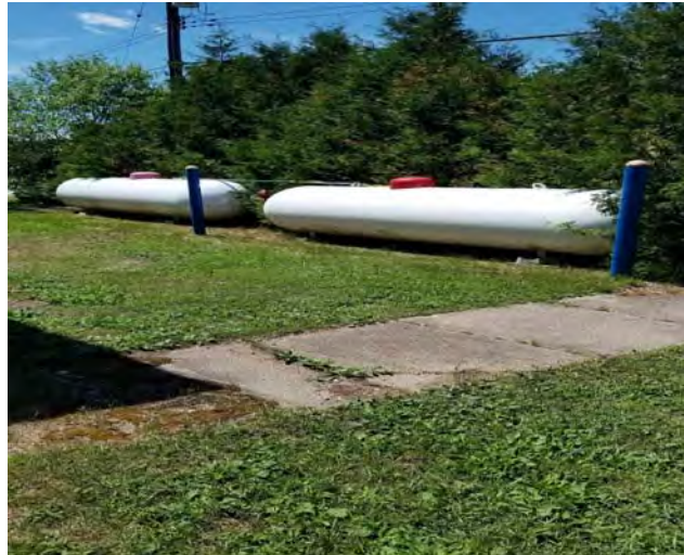
PHOTO OF PROPANE TANK
