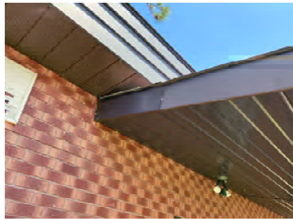
ES002 - Exterior Overhang at Municipal Building
