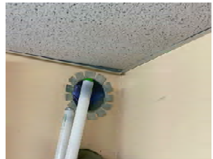
INT090 - Storage and Mechanical Room Thru-wall Ventilation
