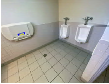
INT145 - Male Washroom Fixtures
