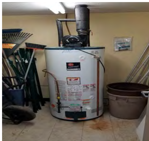
PHOTO OF DOMESTIC HOT WATER HEATER (IN THE COMMUNITY CENTRE)
