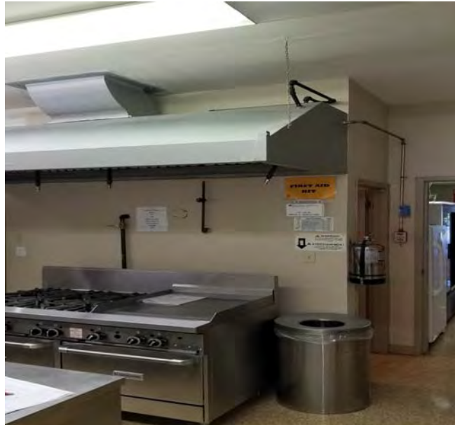
PHOTO OF EXHAUST HOOD (SENIOR'S CLUB KITCHEN)
