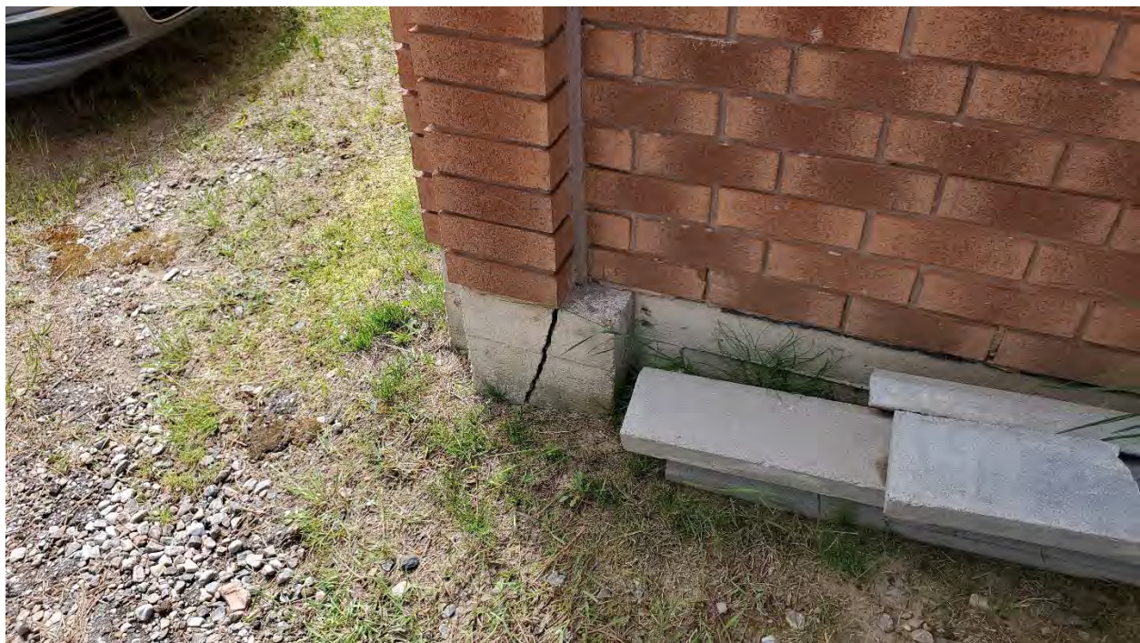
Figure 16: Community Hall Addition: Foundation crack at the northeast corner.
