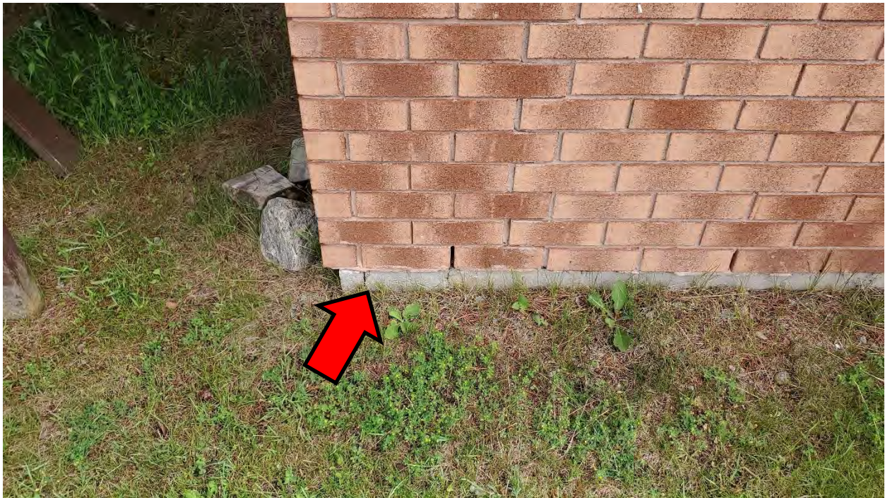
Figure 8: Municipal Office: Southwest corner. Crack in foundation wall.
