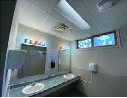
INT138 - Female Washroom Sinks
