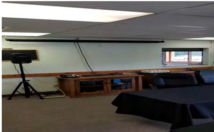
EXISTING LOCAL SOUND SYSTEM AT THE SENIOR GAME ROOM
