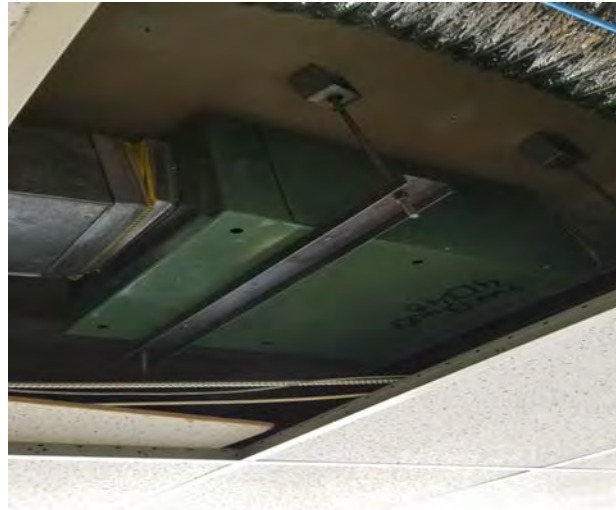
PHOTO OF EXHAUST FAN (IN CEILING OF SENIOR'S CLUB)
