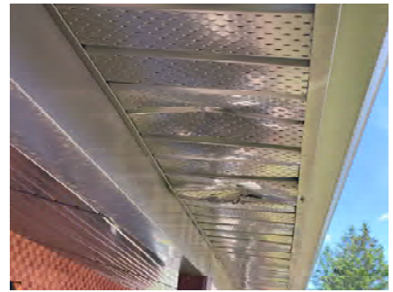
ES006 - Exterior Overhang Soffit Damage
