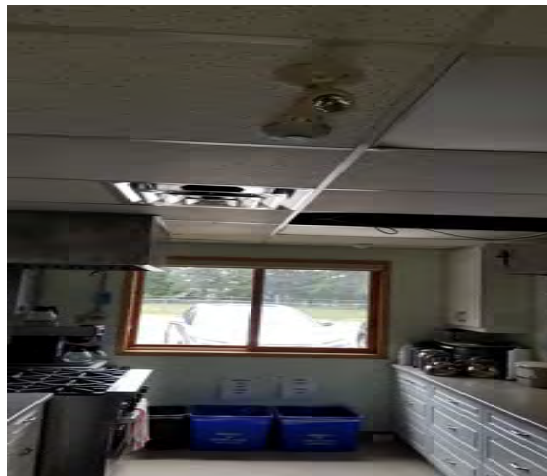
PHOTO OF EXHAUST HOOD (IN THE SENIOR'S CLUB KITCHEN)
