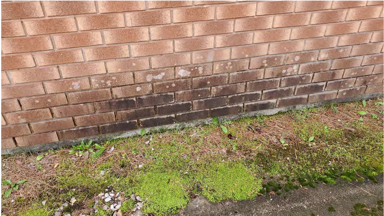
Figure 9: Municipal Office: Deteriorated mortar on the west elevation.
