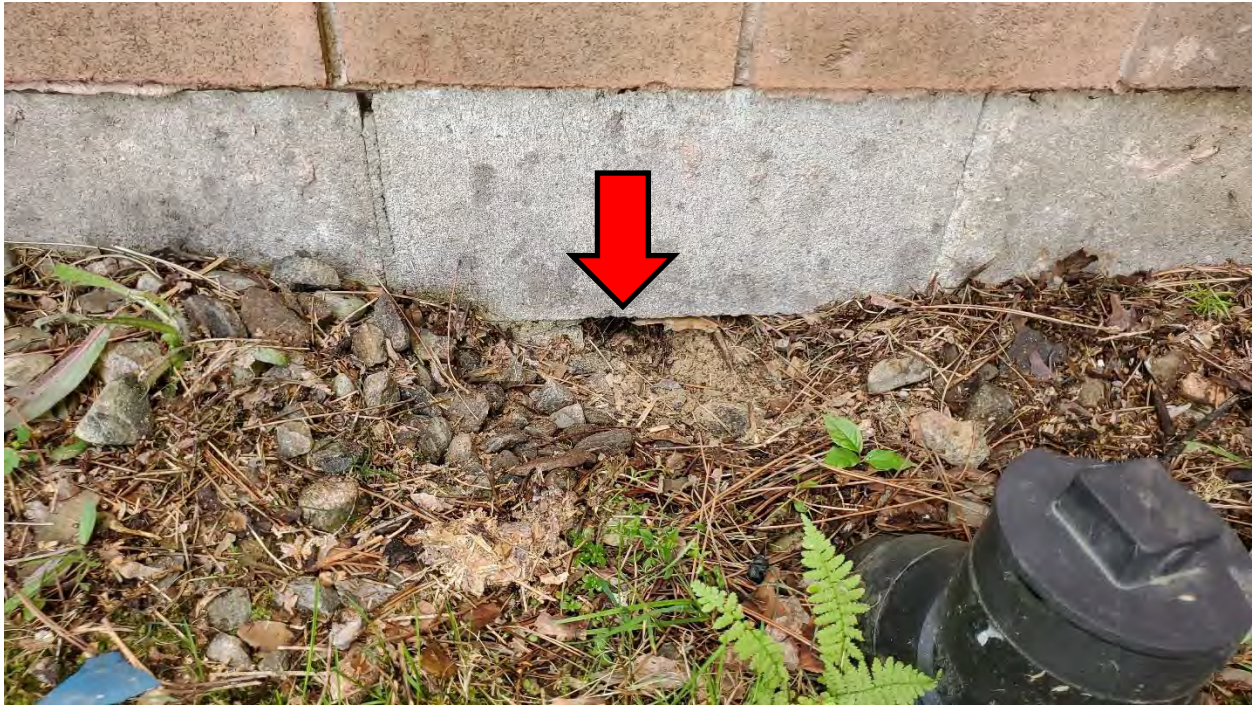
Figure 21: Electrical Room Addition: Hole in the foundation wall on the west elevation of the Electrical Room.
