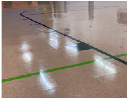
INT040 - Gymnasium typical floor finish
