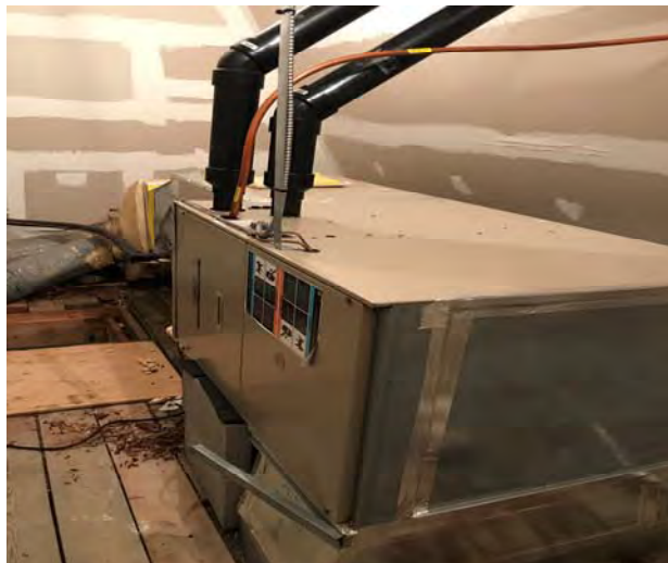
PHOTO OF FURNACE (IN THE ATTIC SPACE OF OFFICE CORRIDOR)
