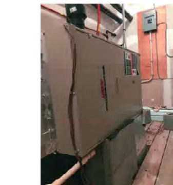
INT116 - Municipal Office Mechanical Room above Corridor
