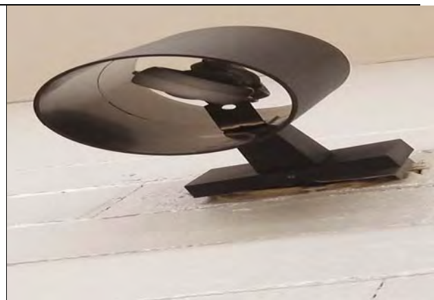
Existing incandescent light fixture at the Gym
