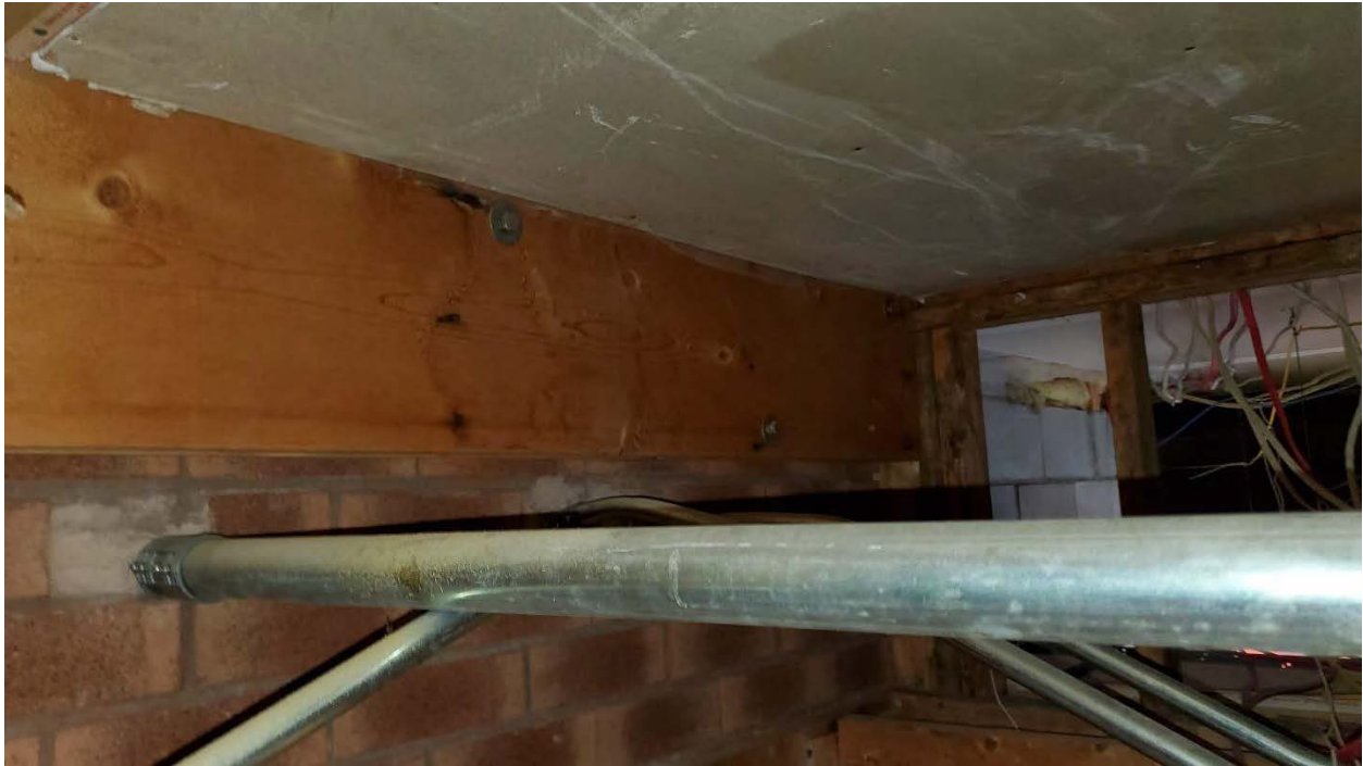
Figure 19: Electrical Room Addition: Wood ledger board bolted to brick cladding in the Electrical Room.
