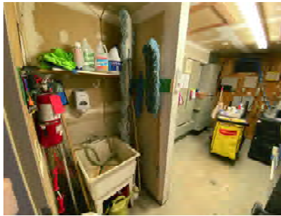
INT022 - Electrical Room Overview looking West
