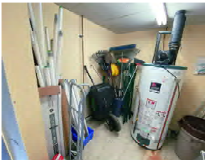
INT089 - Storage and Mechanical Room Hot Water Tank
