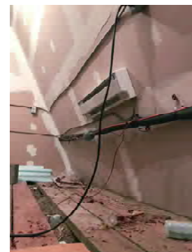
INT117 - Municipal Office Mechanical Room above Corridor Heater
