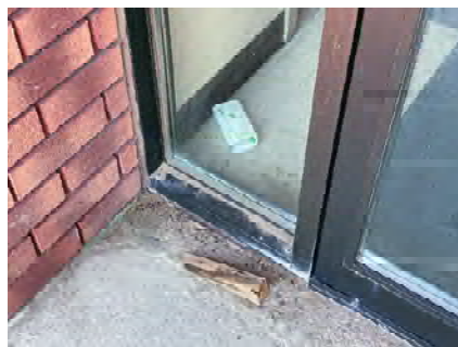
EX035 - Community Hall North Exit Door Sill
