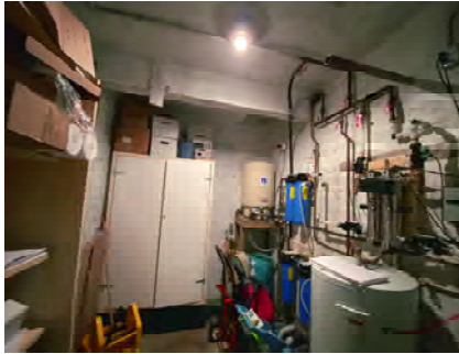
INT149 - Mechanical Room
