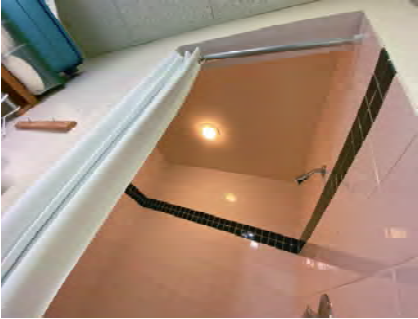
INT80 - Kitchen Storage Shower Ceiling
