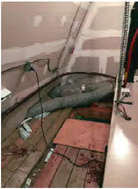
INT118 - Mechanical Room above Corridor Access Hatch
