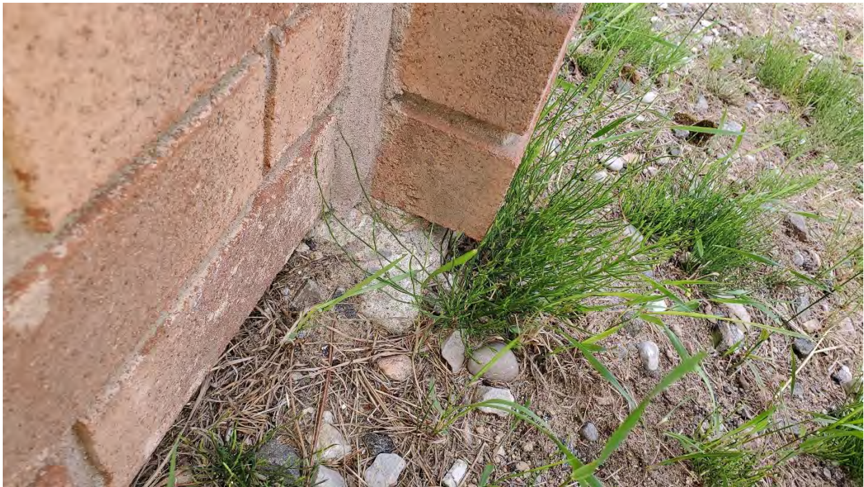
Figure 18: Community Hall Addition: Excessive brick projection beyond the foundation wall on the west elevation.
