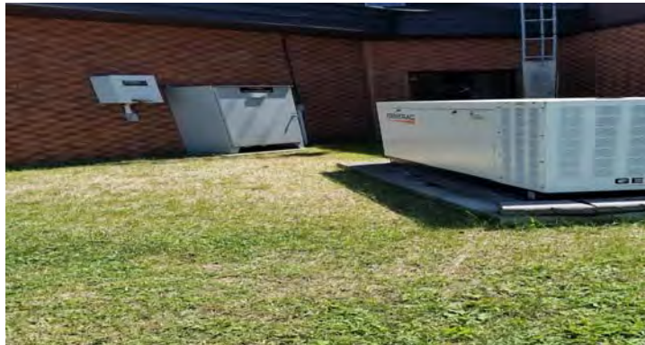
EXISTING OUTDOOR GENERATOR AND AUTOMATIC TRANSFER SWITCH
