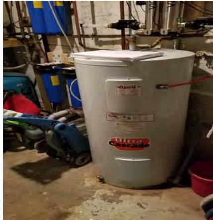
PICTURE OF HOT WATER HEATER
