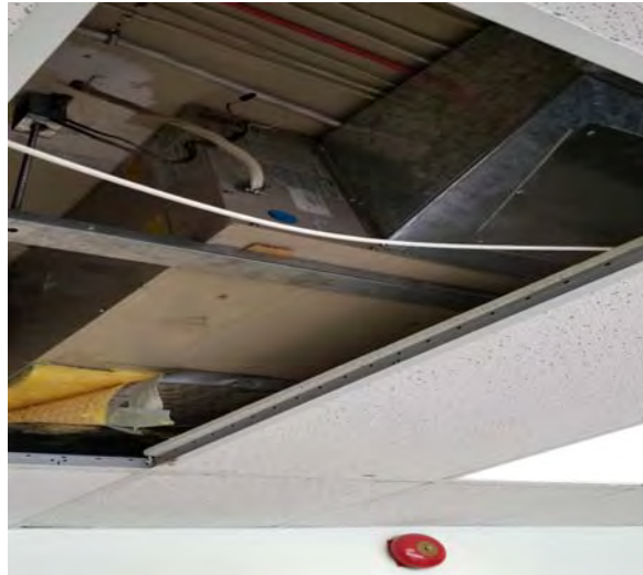
PHOTO OF FAN COIL
