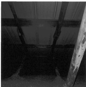
Photograph 19: Metal truss plates dislodged from adjacent trusses
