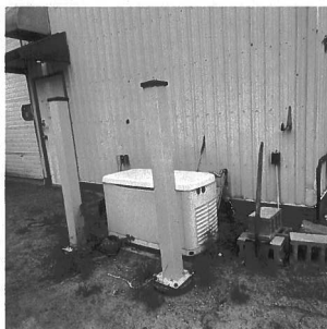
Photograph 8: Emergency generator adjacent to building
