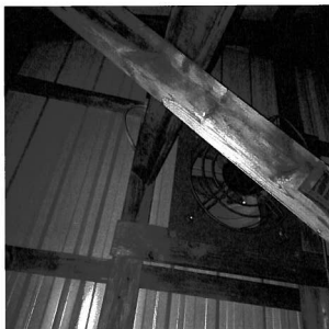
Photograph 25: Existing attic exhaust fan
