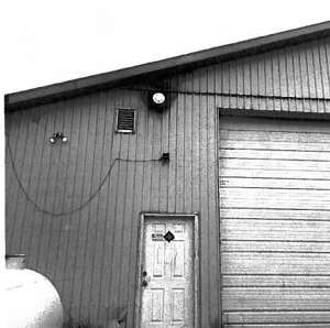
Photograph 21: Exhaust damage to steel siding
