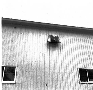
Photograph 22: Vent impact damage
